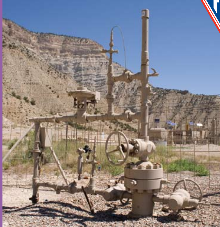
Utilizing new technology pioneered by Ferguson Beaugard, natural gas powerhouses thrive in the rugged Piceance Basin
