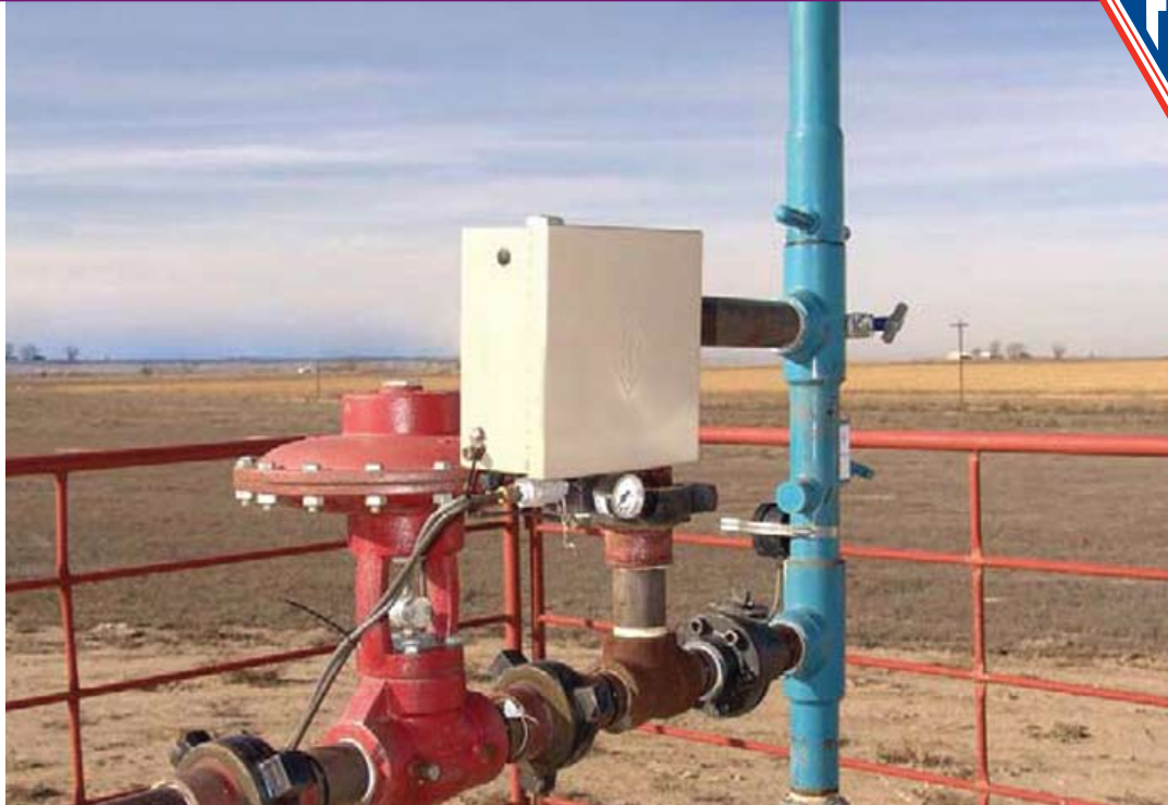
Once a Ferguson Beauregard Two-Stage Plunger Lift System was installed, the well production increased 27 mcf/day
