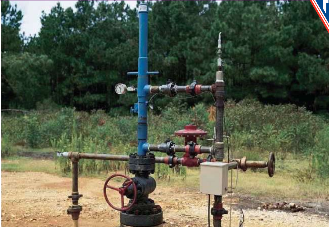
Injection gas decreased by nearly 50% and a 20% to 40% increase in gas production was realized.
