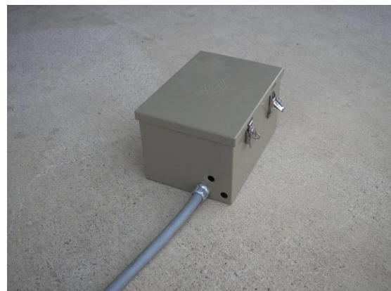
Figure 2.11: Electronic Controller Box
