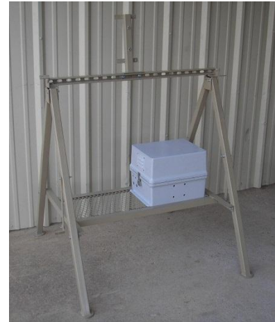
Figure 2.10: Battery Enclosure Mounting
